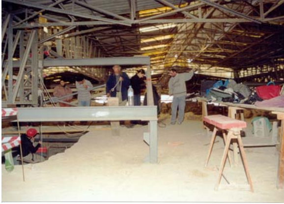
Figure 3. The monuments protective roof cover and the field work area. In the left foreground the fireman charging shot holes in a transmitting shaft.
